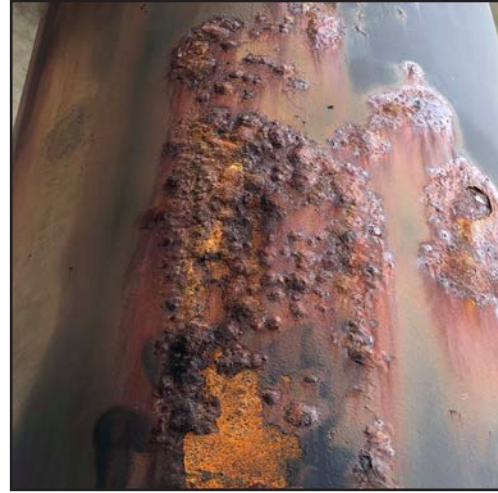
Example image of a pile featuring a loosely adhering corrosion prevention coating that would require removal.
