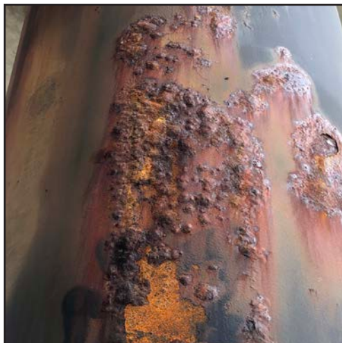
Example image of a pile featuring a loosely adhering corrosion prevention coating that would require removal.
