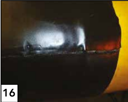
16 A bead of extruded butyl rubber is visible at the edge of the sleeve.
