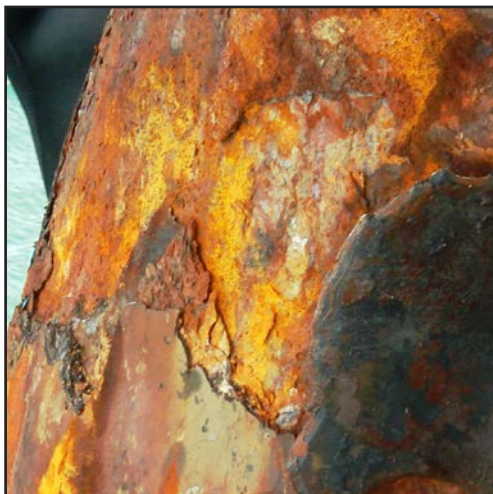
Example image of a pile featuring loose corrosion that would require removal.
